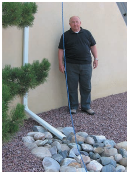
The Church of the Holy Spirit has also installed an energy-efficient drainage system along with other renovations including energy-efficient lighting and lighting, and new heating and cooling systems. Fr. Perkins noted that the renovations were undertaken with an eye to the future of the parish, and they are already benefiting from the savings.
